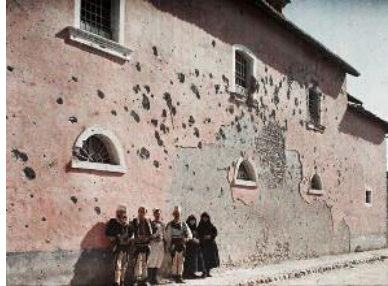
Figure 15 Franciscan Church in Shkoder. The walls show the damage done during the war. Today it is restored
