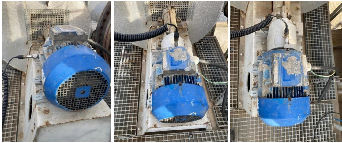
Figure 3.4 Horizontal, Vertical, and Axial Measurement of the Front Bearing of the Motor
