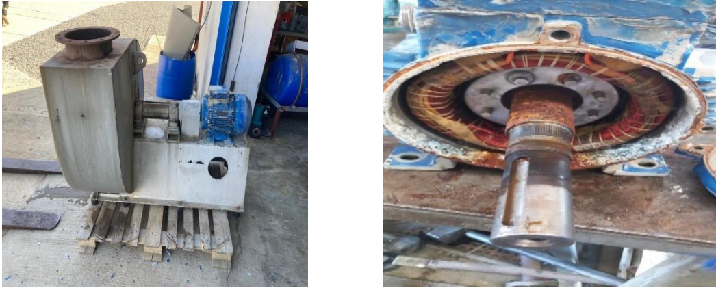
Figure 3.8 Dismantling and Maintenance of the Flue Gas Fan Motor in the Maintenance Workshop
