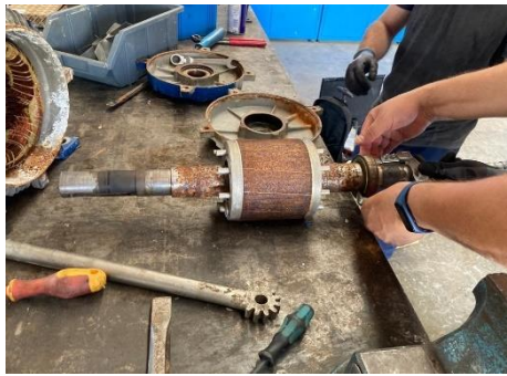
Figure 3.9 Flue Gas Fan Motor Rotor Corrosion
